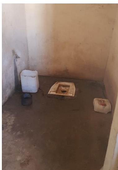
Poor sanitary facilities
