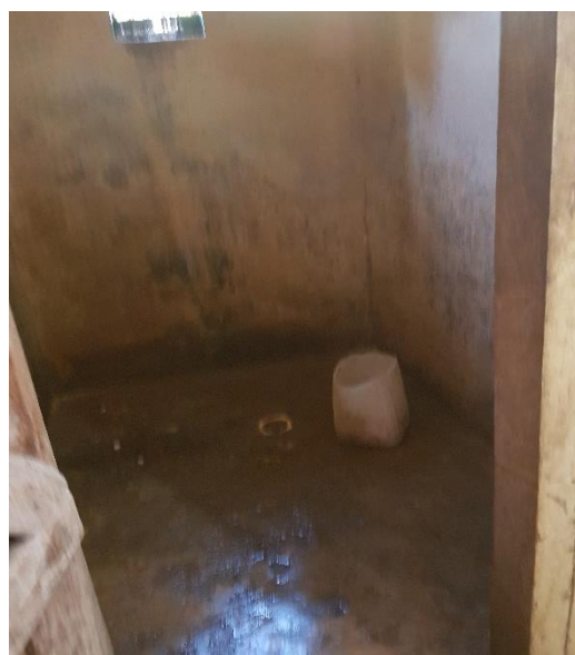
Very poor sanitary facility at the Prisons
